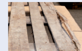
Stringer, partially or fully fractured board
